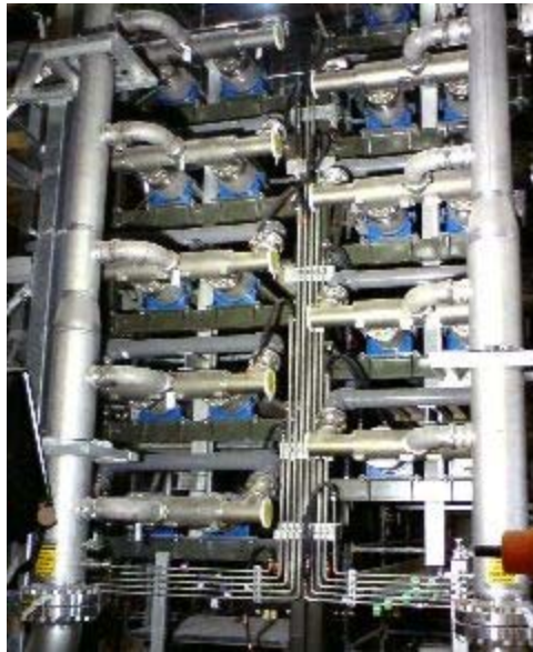
Figure 3: DWEER rack in Sydney, designed to handle 2 Sydney trains or a max. capacity of 41,640 m 3 /d (10 MGD).
