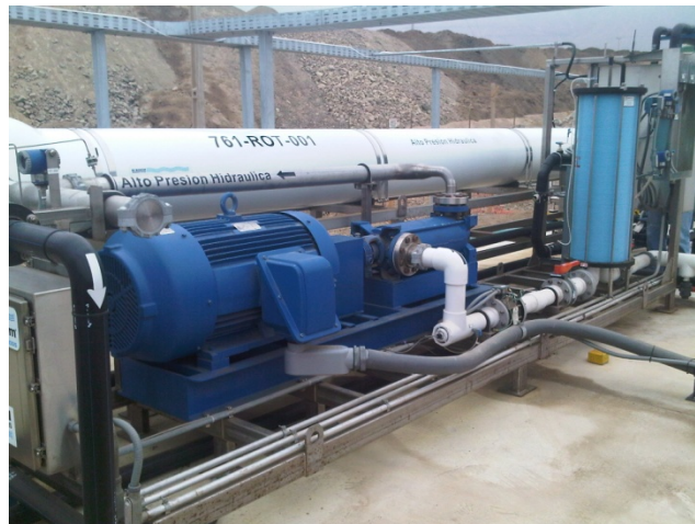
Figure 4: Phase 1 Seawater RO System
