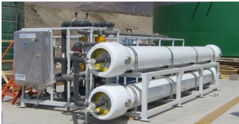
Figure 5: Phase 2 Seawater RO System
