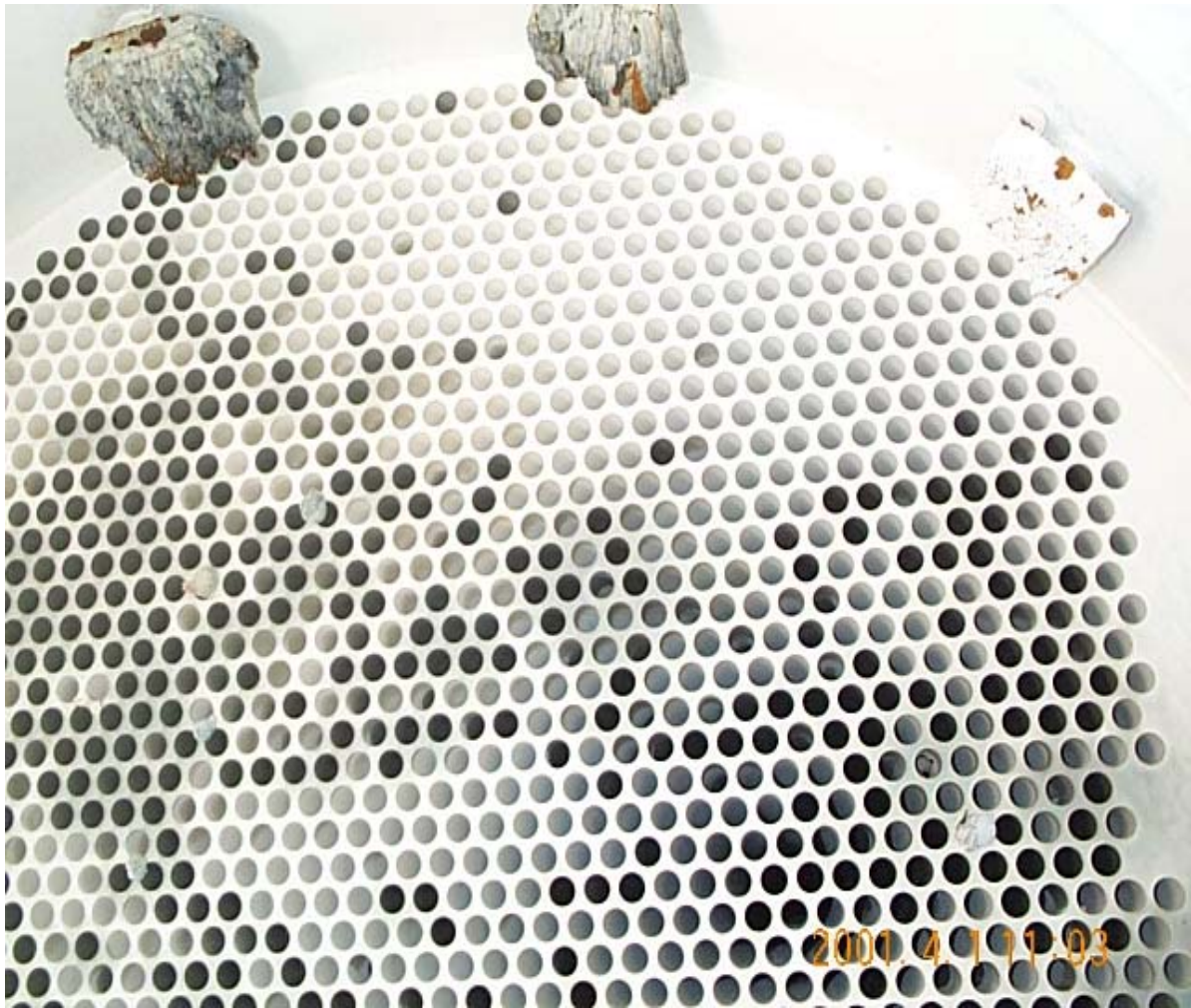
Figure # 2 Anodes at the upper side of a waterbox.
