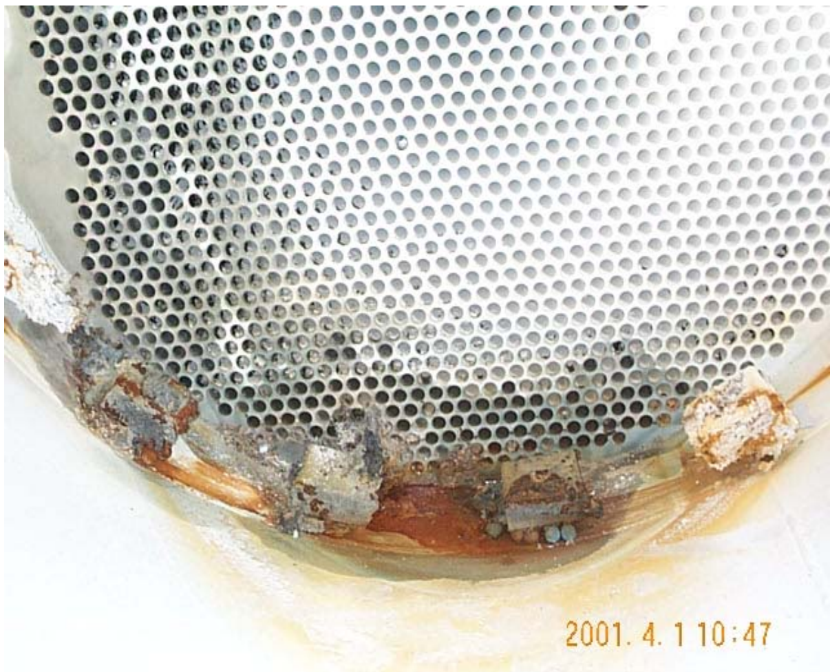
Figure # 1 Anodes of the lowerside of a waterbox
